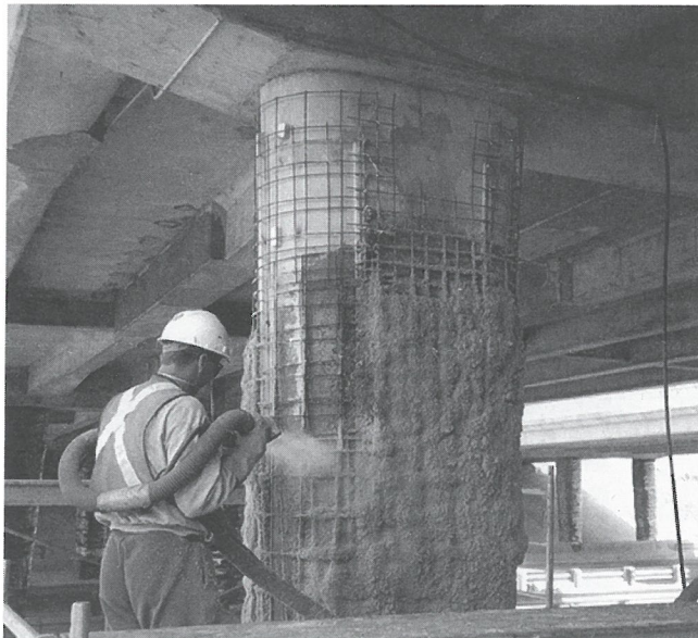
Application of cellulose fibre electrolyte media to bridge columns for Electromechanical Chloride Extraction (ECE) Regina, SK.
